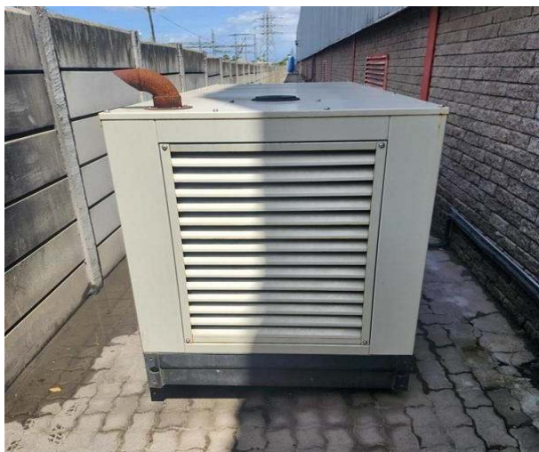
Generator outside admin building
