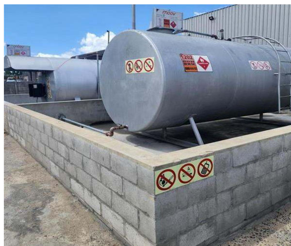
Bunded tank (large)
