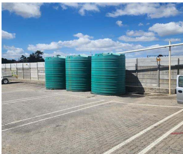
On site water storage
