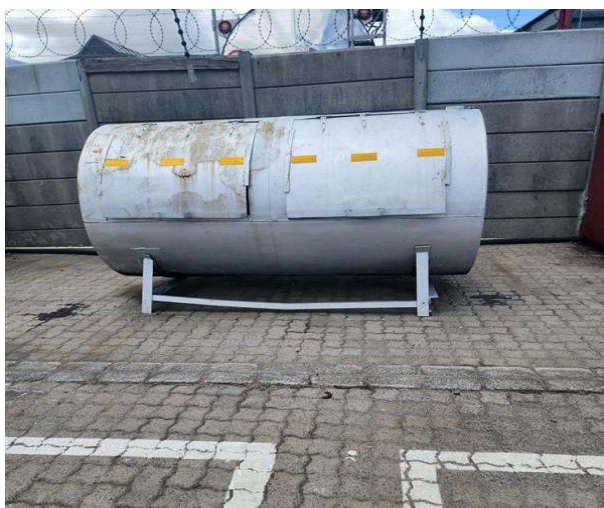
Storage area, empty storage vessel
