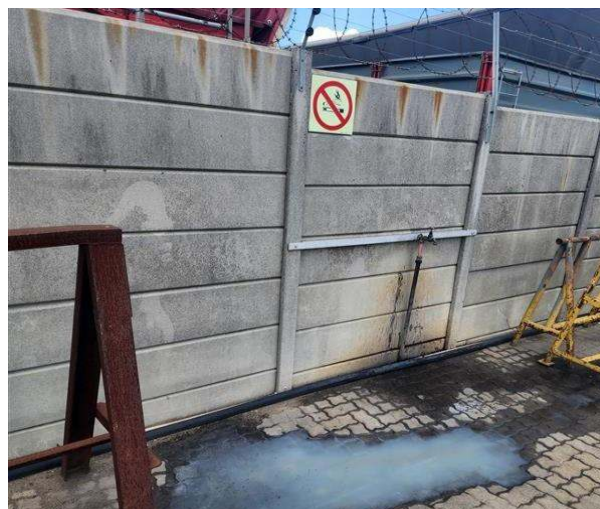
Municipal water at wash bay
