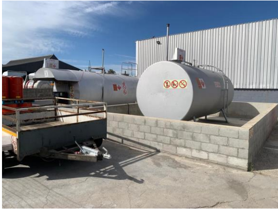
PHOTO 6: View of the two existing tanks housed within a bund.
